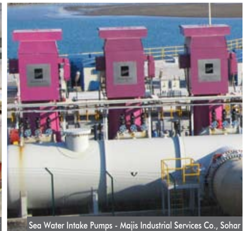
Sea Water Intake Pumps - Majis Industrial Services Co., Sohar
